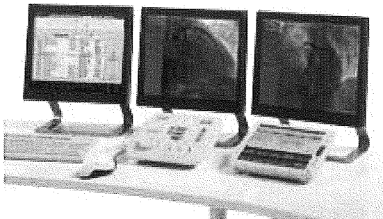
LCD monitors in the control room
